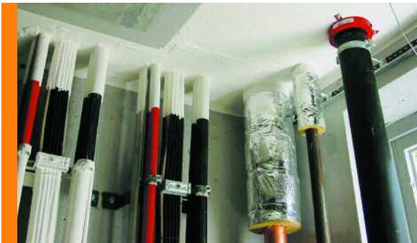
PYRO-SAFE Universalschott COMBI S90 als Deckenschott PYRO-SAFE Universal Bulkhead COMBI S90 as a ceiling penetration seal
